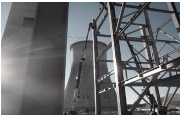
Construction of the boiler structure with a cooling tower in the background.
