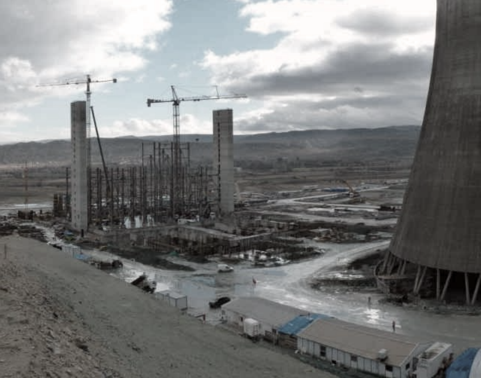
Construction of the boiler structure, the cooling tower height is 115 m, the boiler height is 53 m.
