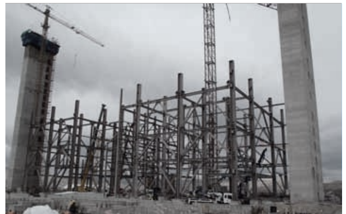
Construction of the boiler structure on which several REMAK air-handling units are placed, these units will stand the highest dynamic load in case of an earthquake.
